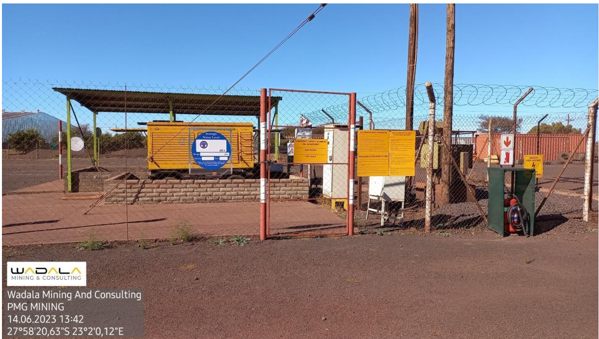
Photo 5: Generator at Workshop.
