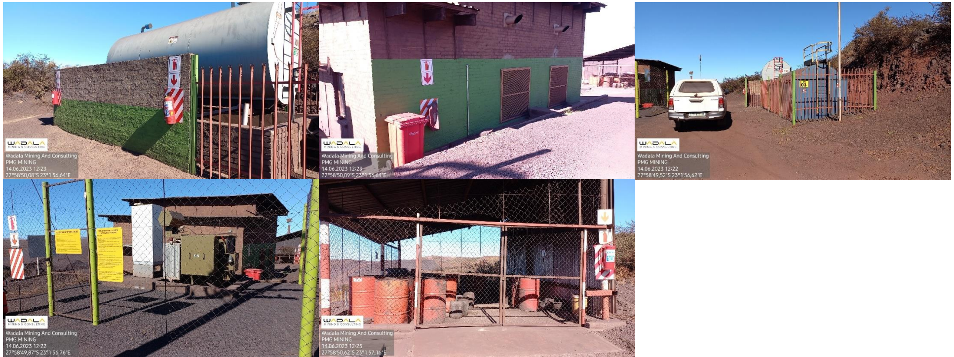
Photo 15: Fuel and Oil storage as well as generator at the Processing Plant.
