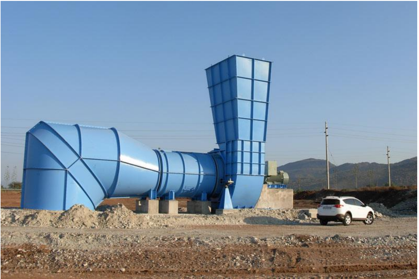
Figure 6-1: A typical ventilation shaft surface infrastructure (Greene Group Consulting Engineers (Pty) Ltd, 2024)
