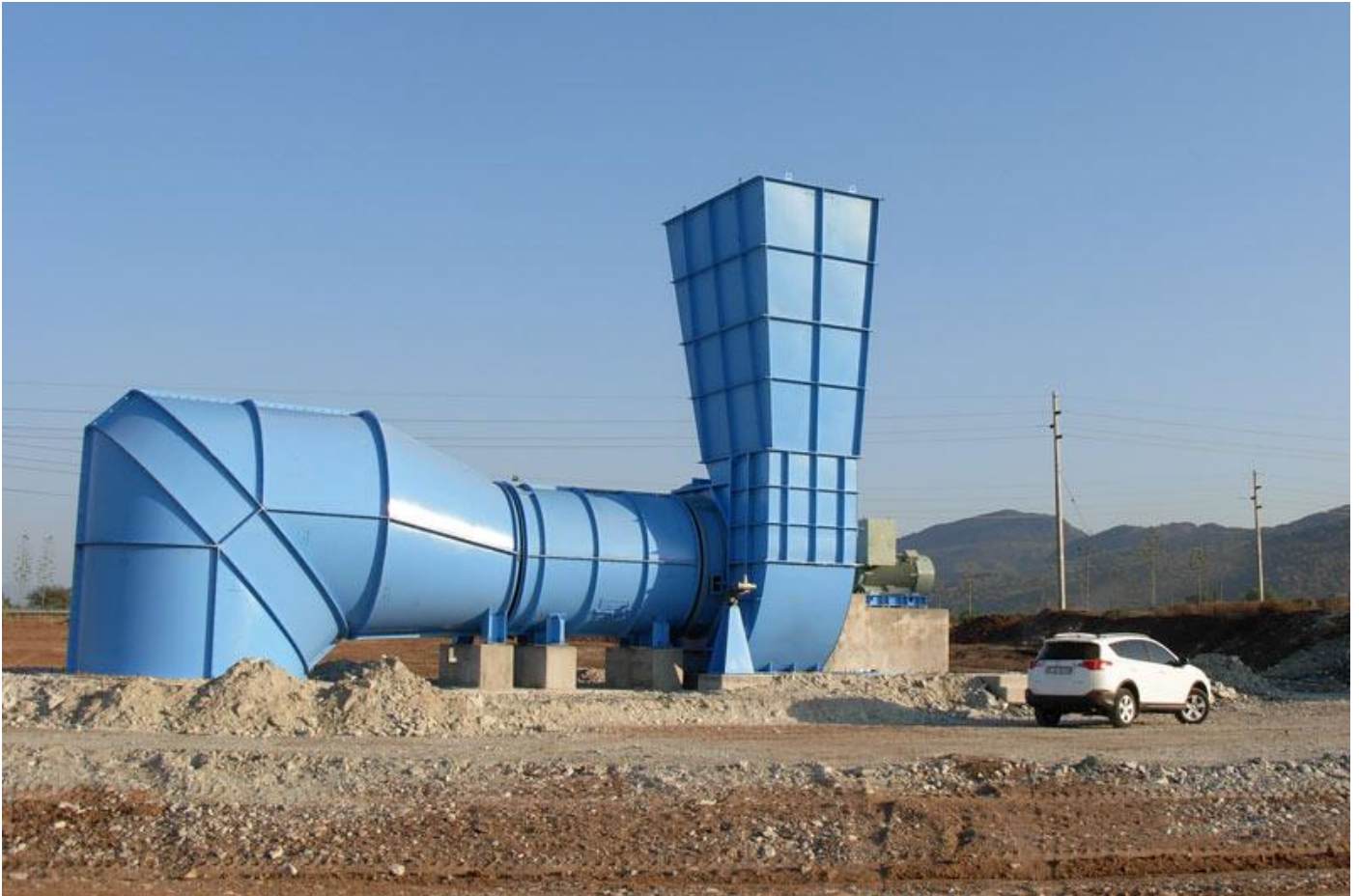
Figure 5-43: A typical ventilation shaft surface infrastructure (Greene Group Consulting Engineers (Pty) Ltd, 2024)
