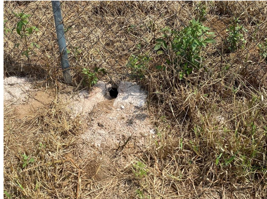
Photo 4: Holes on embankment
