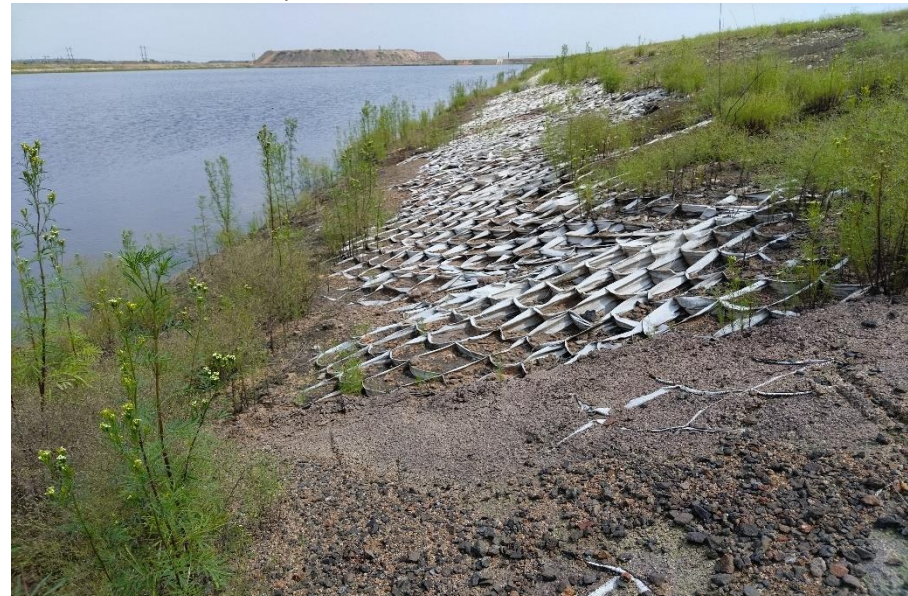
Photo 2: Wall inner slope condition
